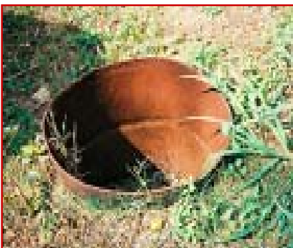
The access to an underground fat trap in a small plant.
