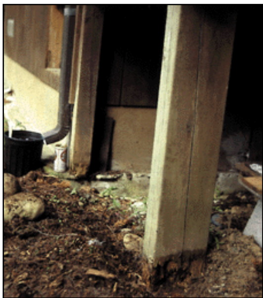
Water damaged wood in contact with the soil. This is a great place to look for moisture ant colonies (photo by Art Antonelli).
